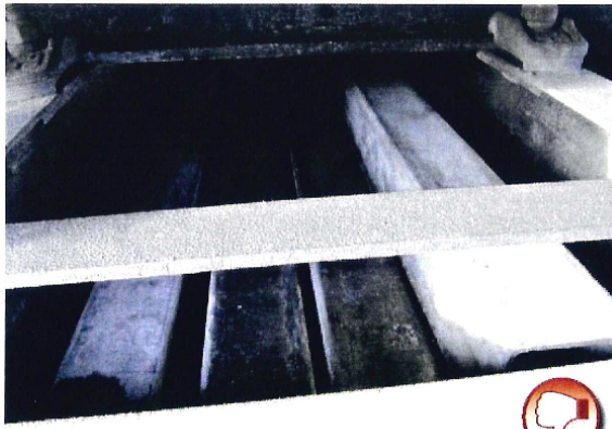
Quantity of additional stanchions Missing additional stanchions
